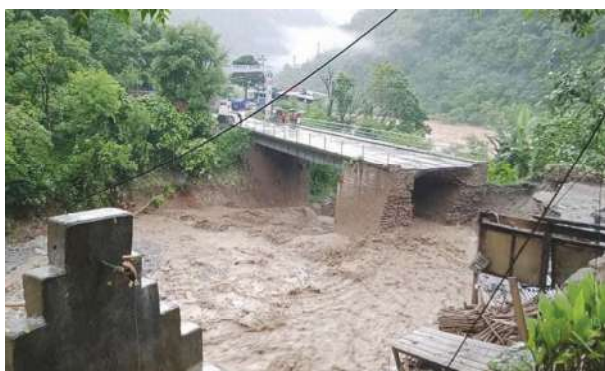
फोटो : Scouring of Abutment backfilling (More coarse grained material) due to peak Flood in Mouwakhola, Dhanding, Source: Online news
