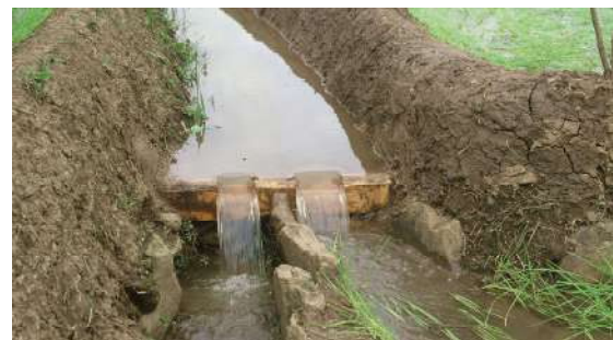
फोटो : Reduction on canal capacity due to growth of vegetation at side slopes and even siltation in bed.
