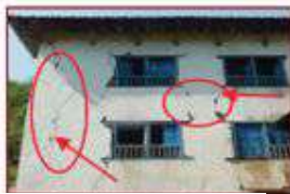
Grade 3 cracks in plastered walls
