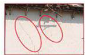
Grade 2 cracks in cement plastered walls
