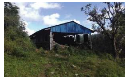
फोटो : Wall Colapsed due to lack of bands from Gorkha Earthquake
