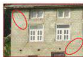
Exposed Masonry Walls having Grade 2 cracks
