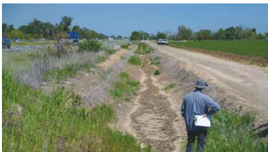
फोटो : Canal not in use due to damage in or failure of lining
