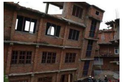
फोटो : Tilting Building by Gorkha Earthquake 2072
