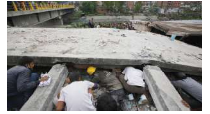
फोटो : Building Collapse due to weak beam column connection in Gorkha Earthquake
