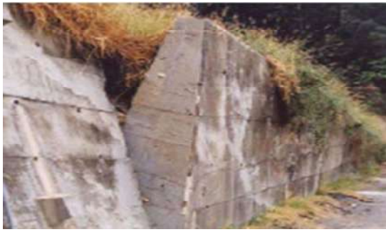
फोटो : Shifting of Concrete Retaining Wall due to excess surcharged load on backfill
