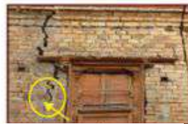
Grade 3 cracks in unplastered walls
