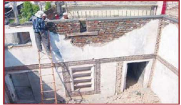
Damaged brick masonry wall being rebuilt to reinstall Rc slab on it
