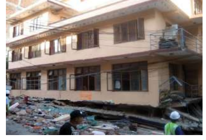
फोटो : Soft Storey Failure from Earthquake
